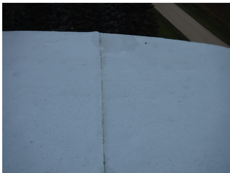
24) The roof coating is in poor condition overall.
