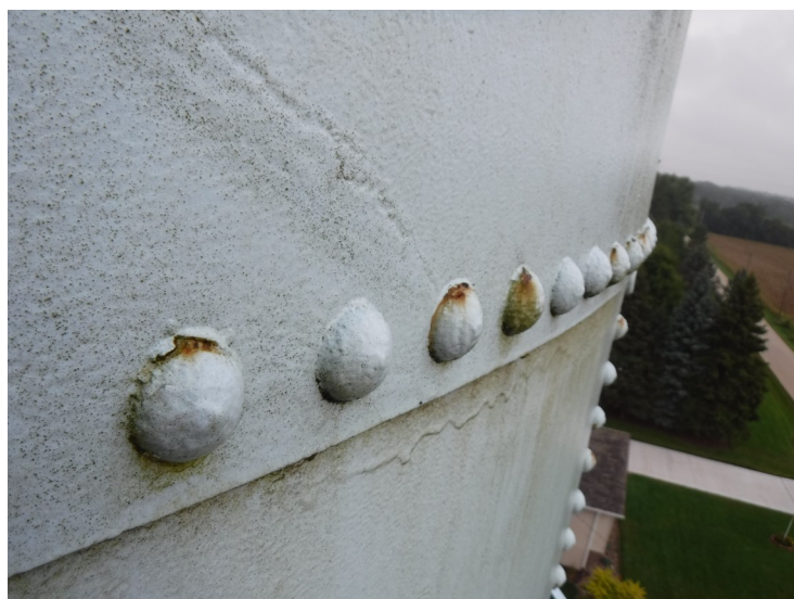
21) Spot coating failures on the sidewall.
