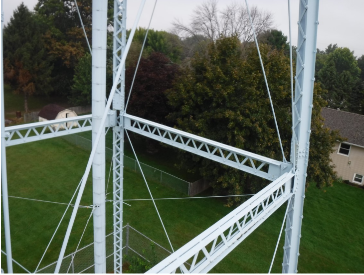
13) The sway rod coating is in fair condition.
