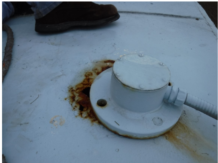
26) Coating failures on the roof. There are small holes through the roof at the penetrations.
