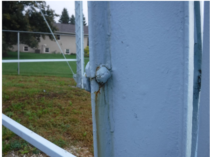
8) The leg coating is in fair condition overall with several spot coating failures.
