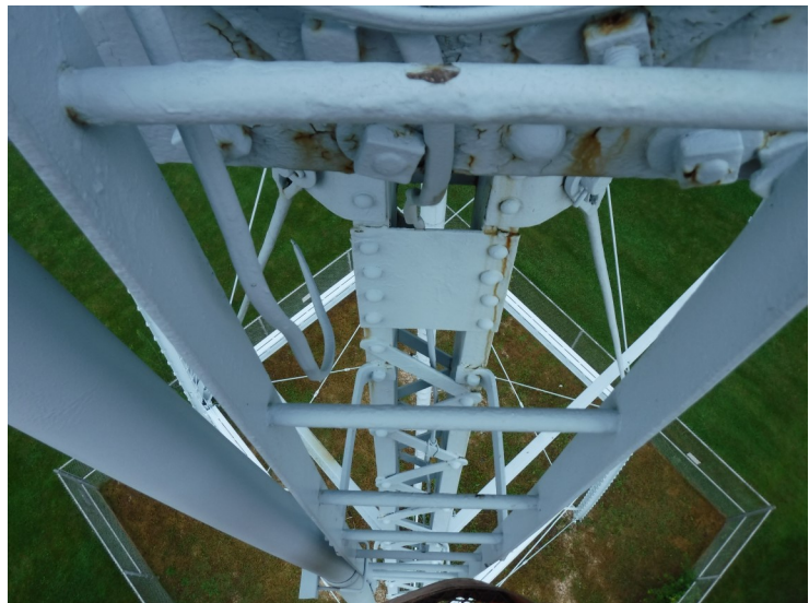
11) The ladder extends down approximately 6 feet from the balcony. The coating is in poor condition.
