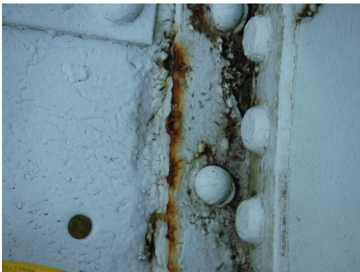
18) Spot coating failures on the balcony.
