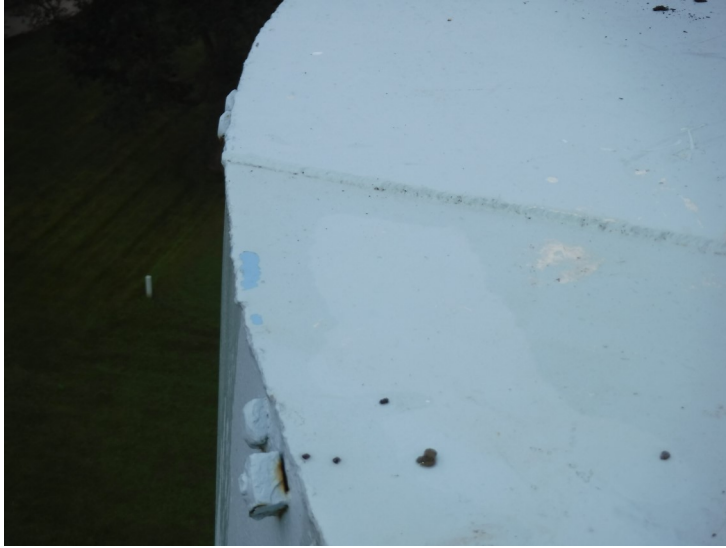
25) Topcoat delamination on the roof.
