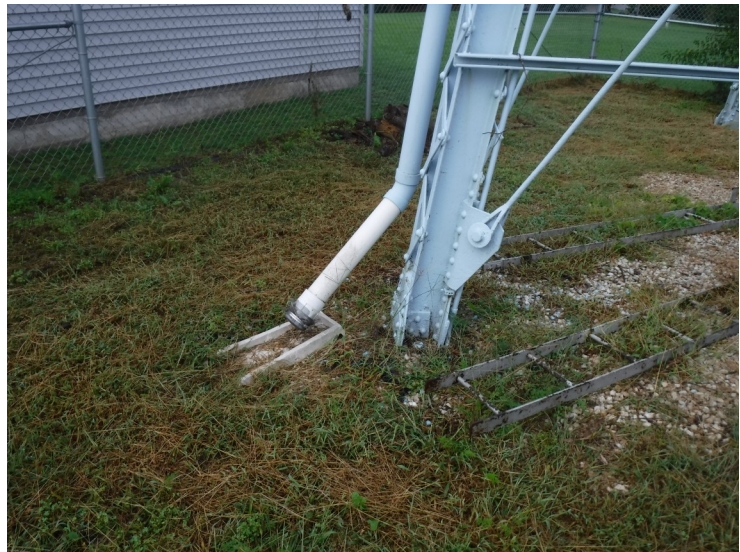
5) The overflow pipe is constructed of PVC. The PVC is in good condition.
