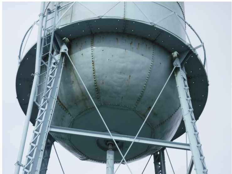
14) The bowl coating is in poor condition.
