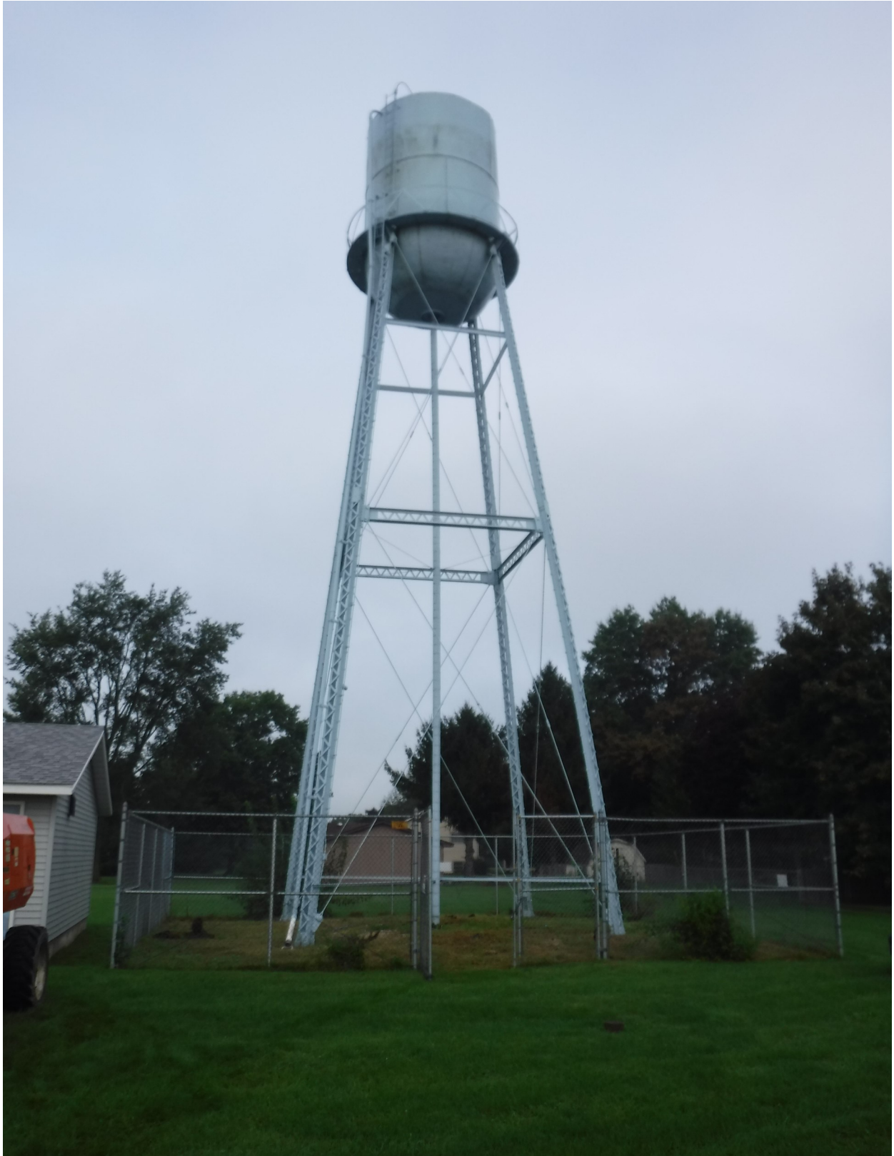
25,000 gallon elevated legged water storage tank located on Buysse Road in Coal Valley, Illinois.
