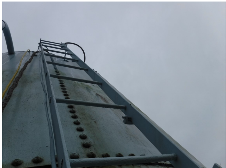
23) The sidewall ladder coating is in poor condition.
