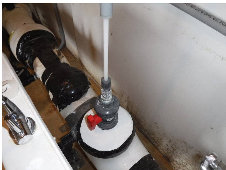
42) The piping is covered in insulation.
