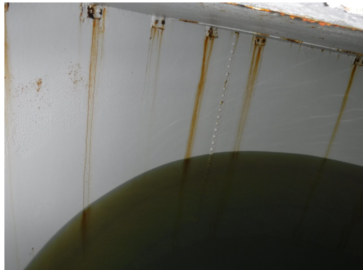
32) Coating failures on the upper sidewall.
