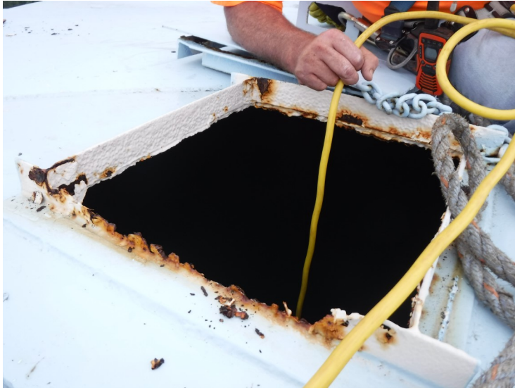
28) The roof hatch neck is severely deteriorated and the cover is no longer attached to the hinge.
