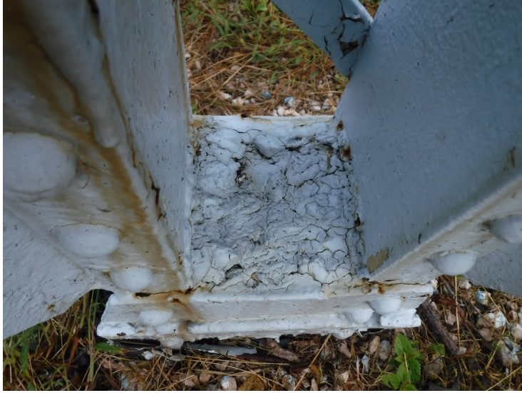
7) There is a build-up of tar that was overcoated in the bottom of the lattice legs.
