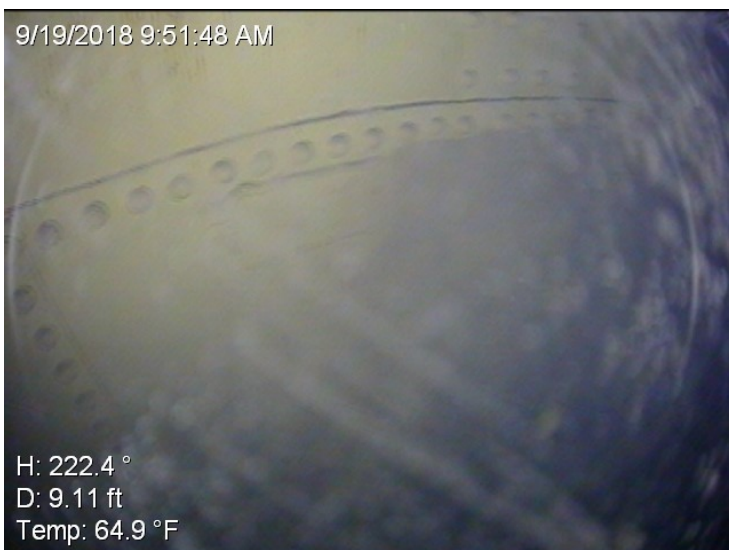
33) Spot coating failures on the sidewall.
