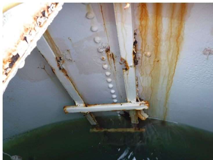
36) The top rungs are missing on the wet interior ladder.
