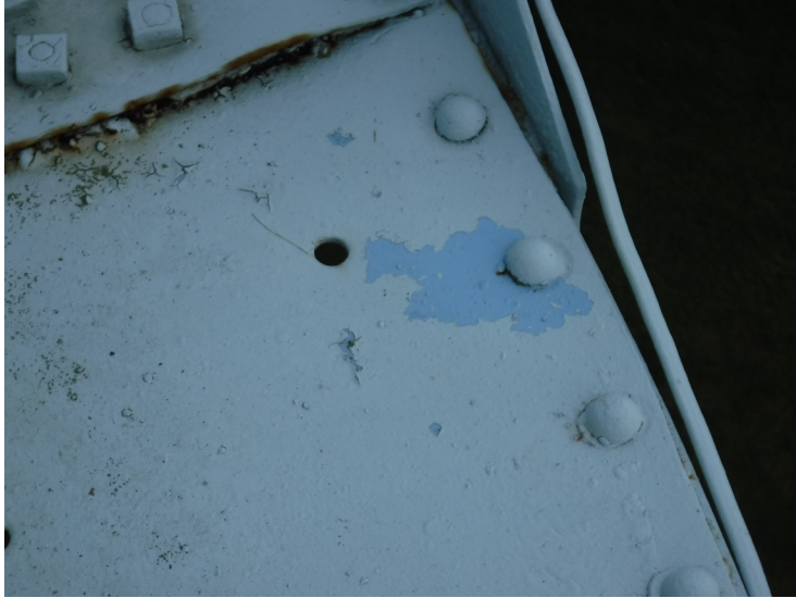
19) Coating delamination on the balcony.
