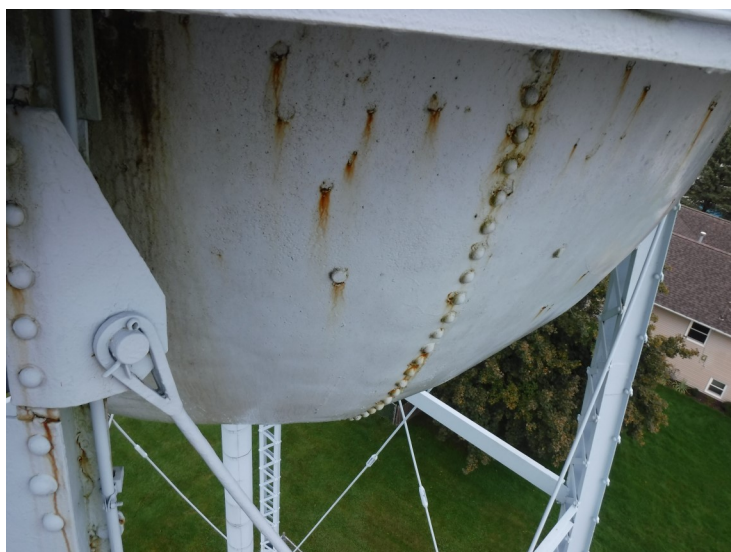
15) Spot coating failures on the bowl.
