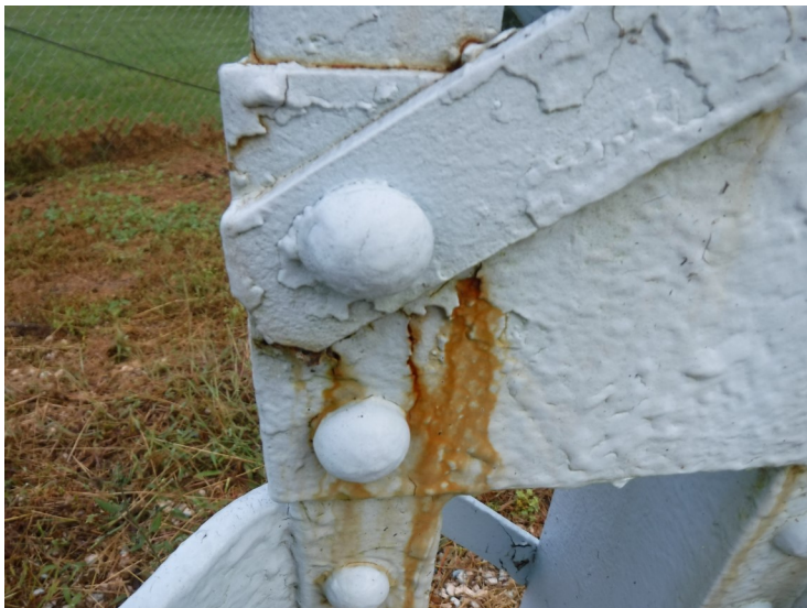
9) Spot coating failures on a leg.
