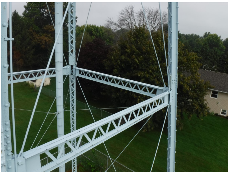
12) The coating on the struts is in fair condition.
