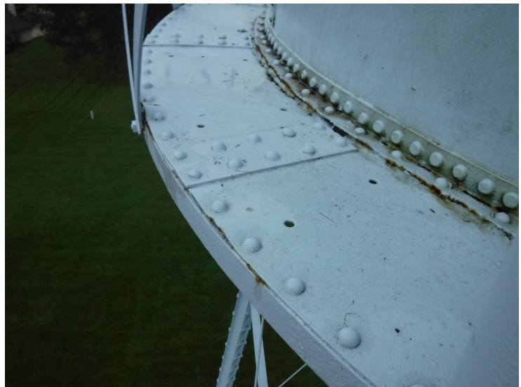
17) The balcony coating is in poor condition. There is no kickplate on the balcony railing.
