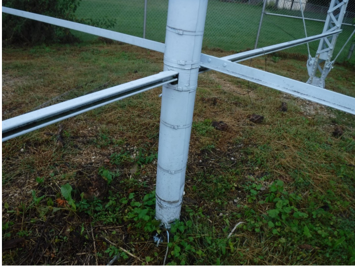
1) The fill/draw pipe routes into the ground.
