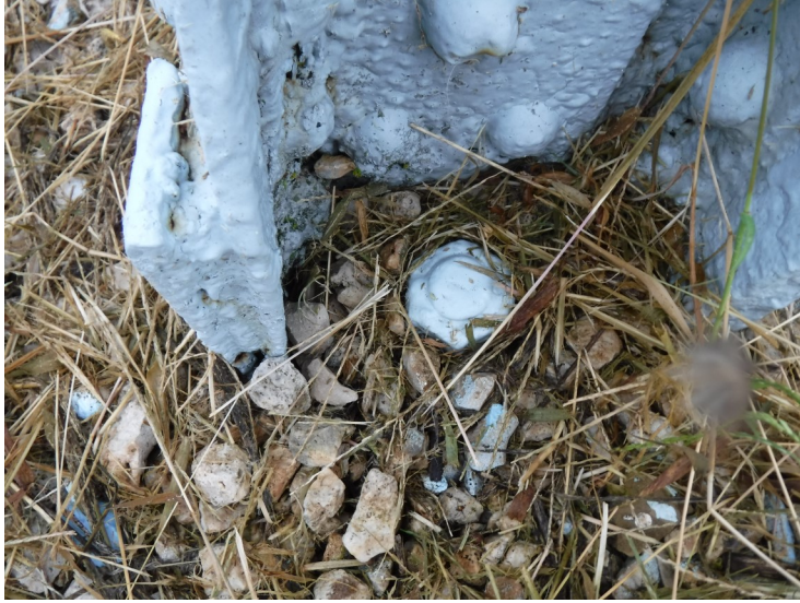
4) The anchor bolts are mostly covered in soil and gravel. The exposed coating is in fair condition.
