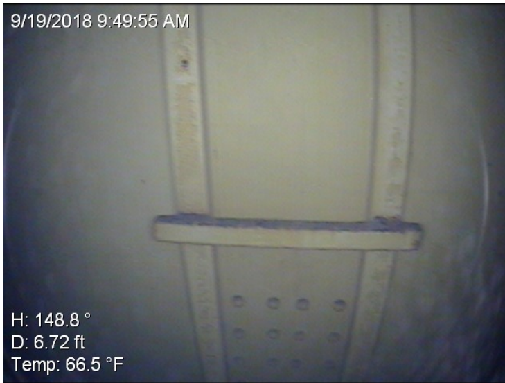
37) Wet interior ladder rung below the high water line.
